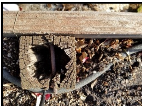
Rotting post—note the exposed bolt
